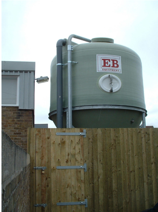
Wood pellet silo for Acomb Library
